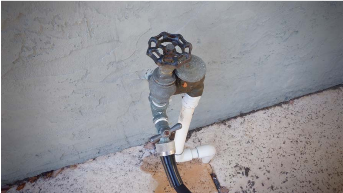
Picture 15 - Pool Water Valve
