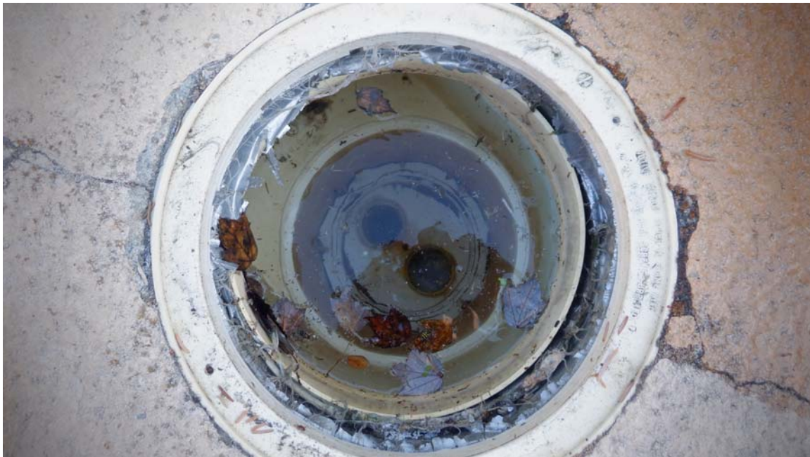
Picture 10 - Float Valve missing in skimmer.
