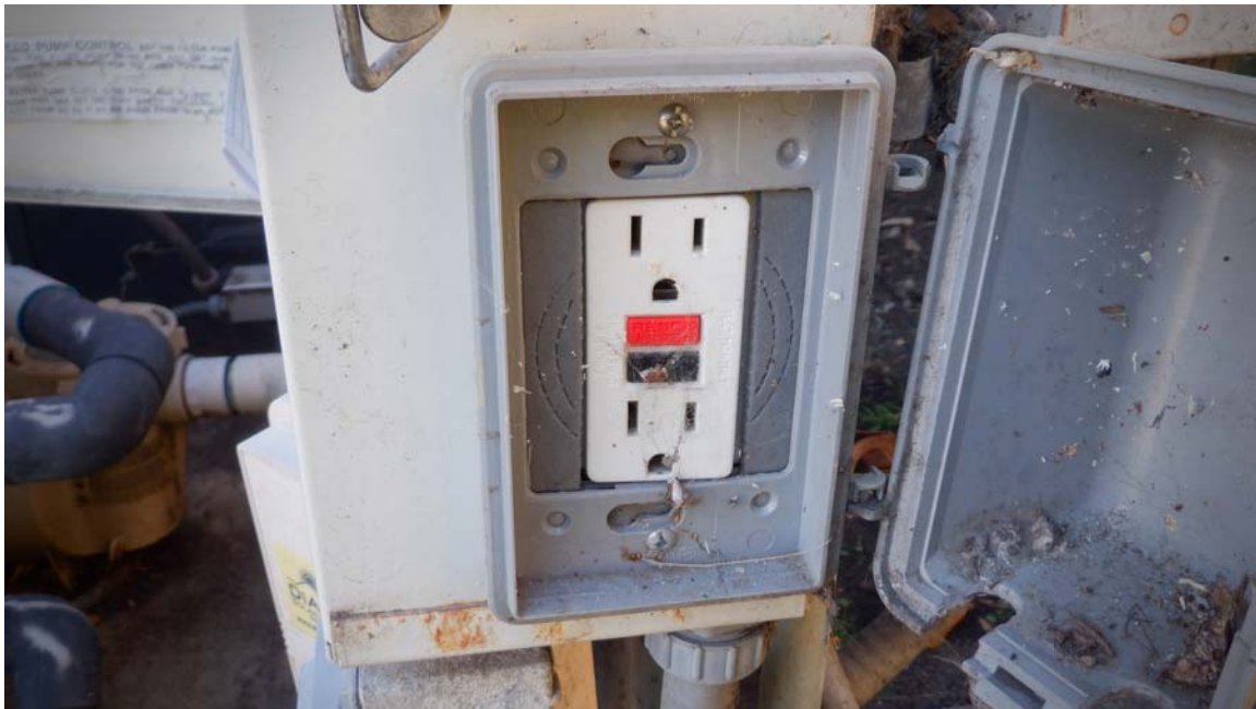
Picture 16 - GFCI Protected Receptacle
