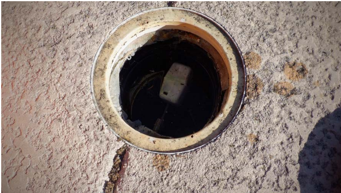
Picture 14 - Pool Water Auto-fill
